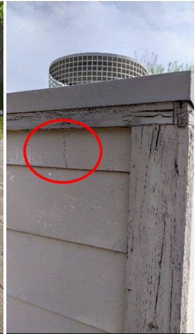
Trim rot/small crack
