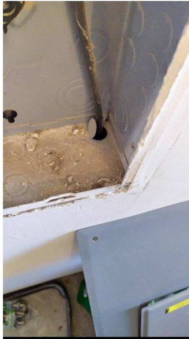
Need cable clamp
