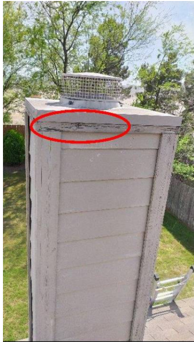
Chimney trim rot
