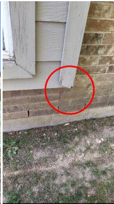
Trim needs paint
