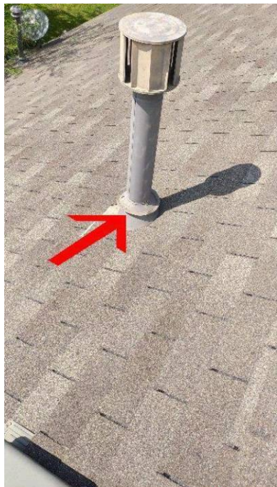
Re-seal storm collar
